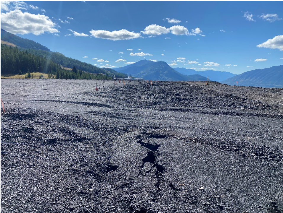
Photo I-3 CCR Dump surficial cracking behind crest. (Looking south – Taken 20 September 2022)
