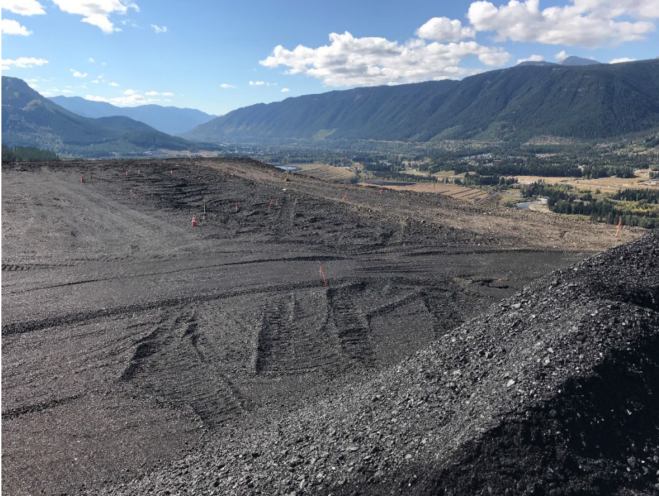
Photo I-13 CCR Dump surficial cracking behind crest. (Looking SW – Taken 20 September 2022)
