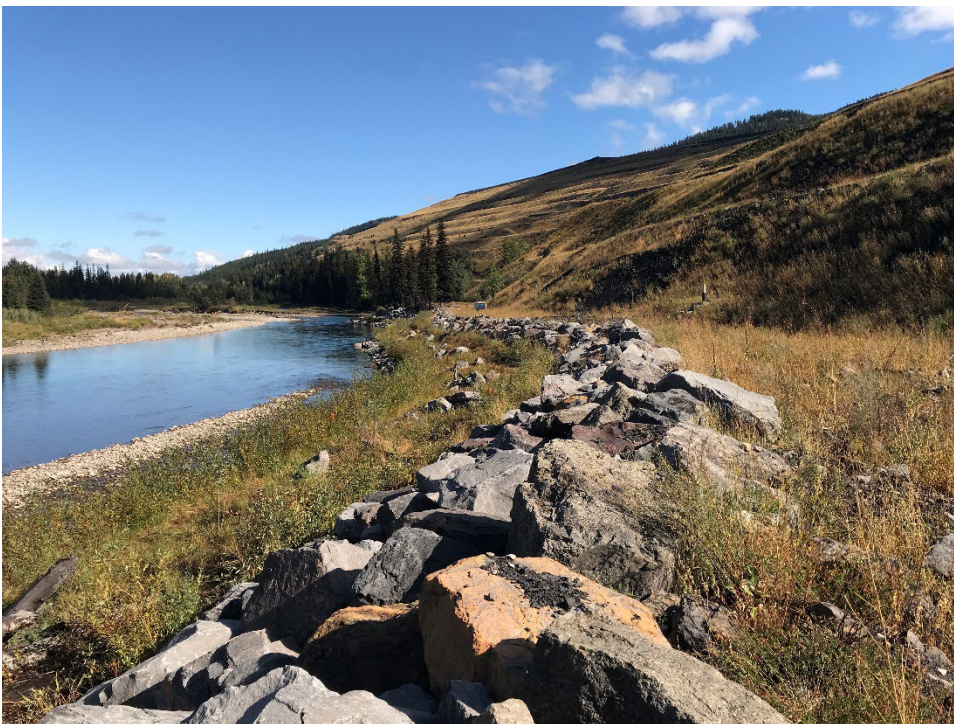
Photo I-2 CCR Dump overview and slope toe along the Elk River with riprap. (Looking NE – Taken 20 September 2022)
