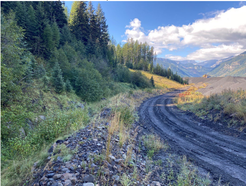
Photo I-10 CCR Dump diversion ditch and Lindsay Drain extension. (Looking west – Taken 20 September 2022)
