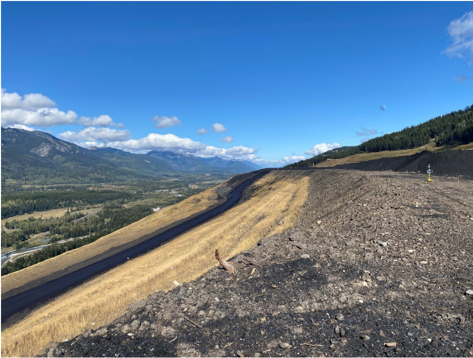
Photo I-17 CCR Dump crest and slope below surficial cracking. (Looking north – Taken 20 September 2022)
