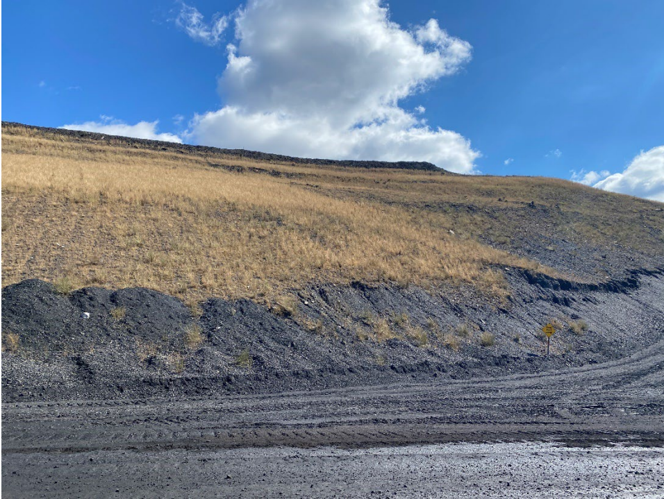
Photo I-19 CCR Dump slope below surficial cracking. (Looking SE – Taken 20 September 2022)
