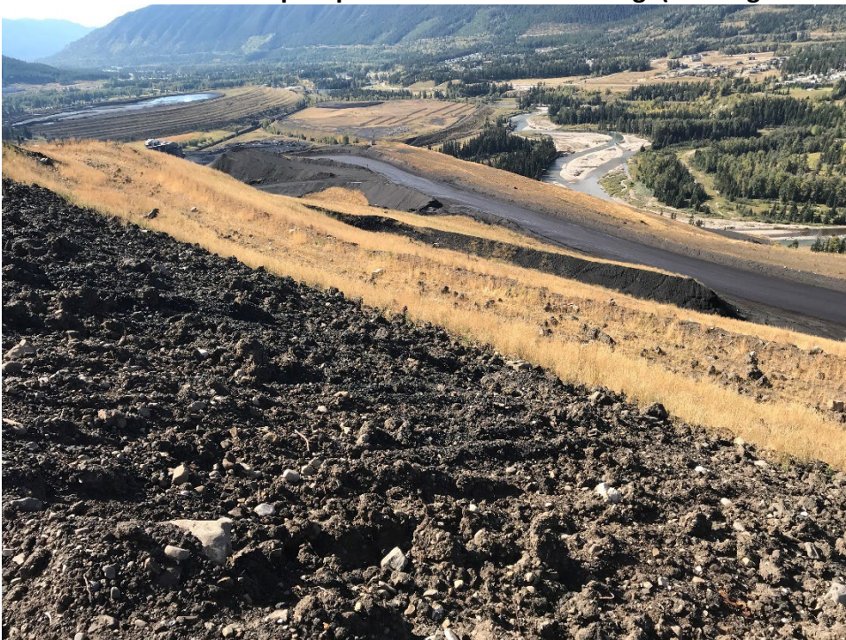
Photo I-18 CCR Dump slope below surficial cracking. (Looking SW – Taken 20 September 2022)
